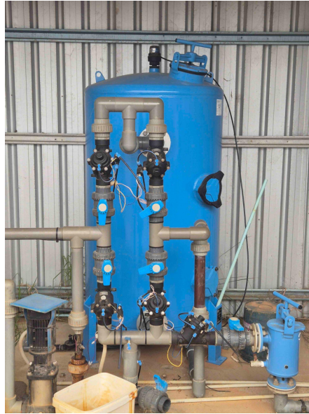
Figure 19. Water filtration unit to treat bore water
