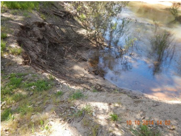
Photograph 13 – View of flood washout, 2014. Photo R.McPherson
